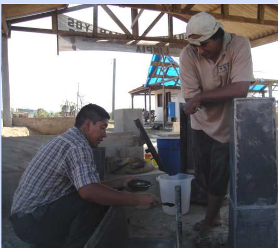
Filter Technicians Felipe Quispe (left) and Angel Perez work together to improve the concrete mix for COBAGUAL's filters (July 2008)
