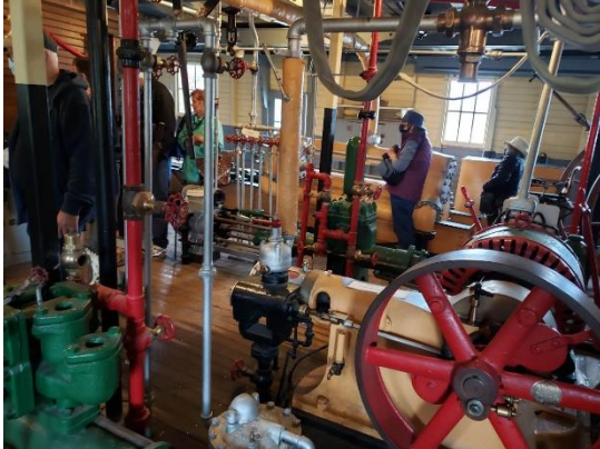
Engine room of the SS Moyie
