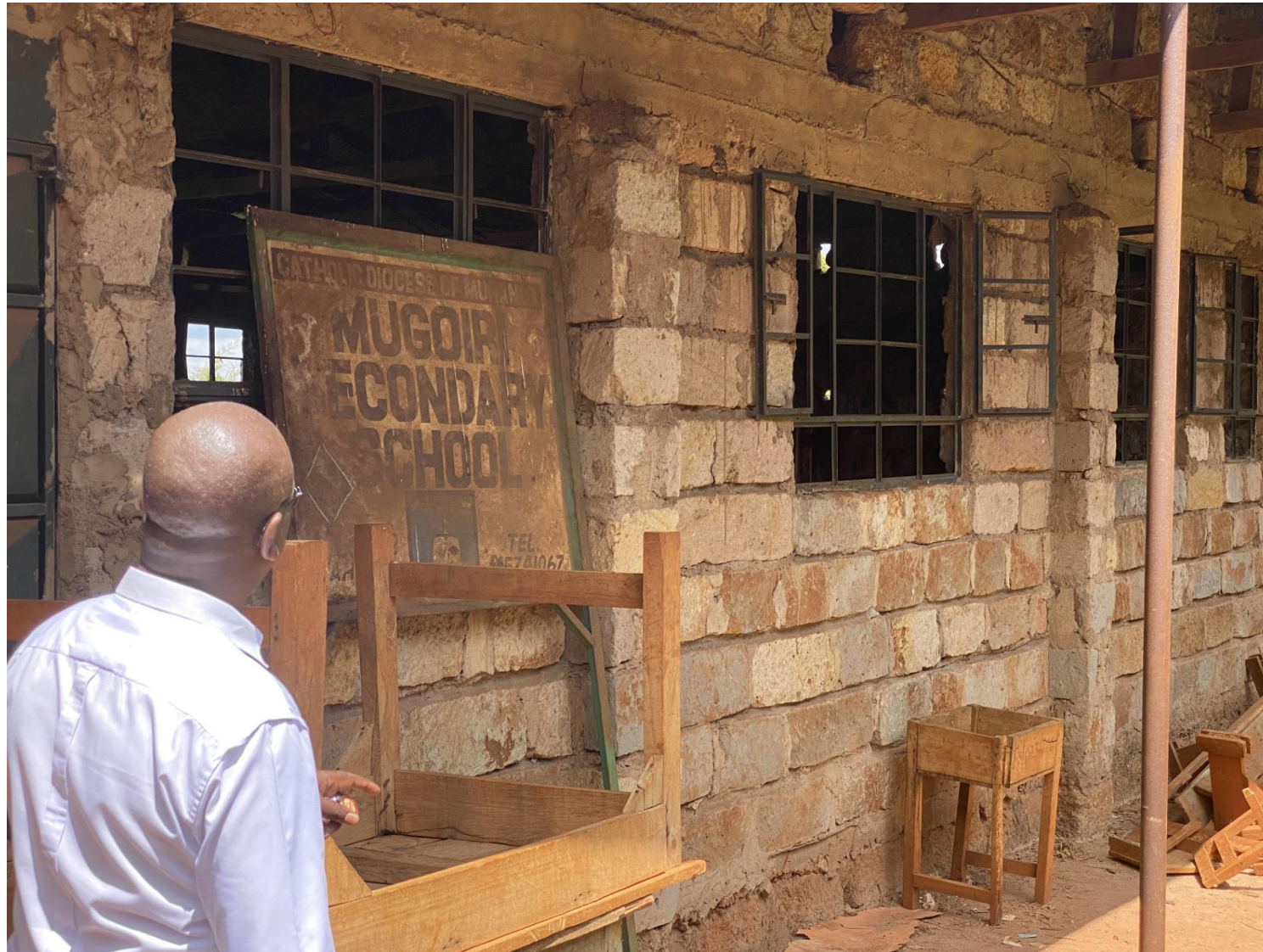
Unfinished classrooms, many students sit on bare concrete floors
