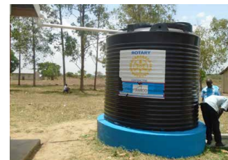
Rainwater harvesting tank
