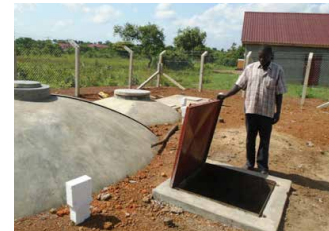
Biogas Conversion tanks
