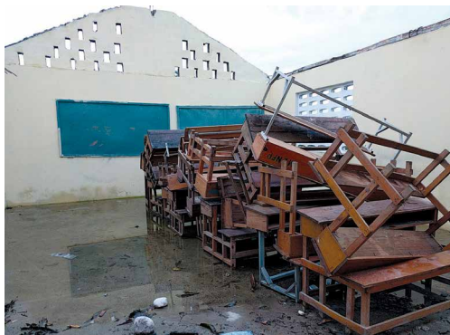
Damage at a Haitian school
