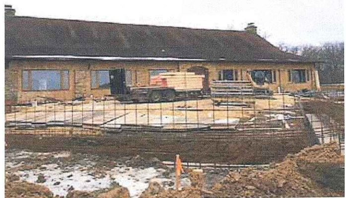
Renovations are underway to give the lodge at Eagle Point Park in Clinton new life for the next 100 years!
