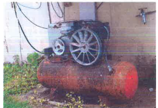
Figure 1. The existing pump system at VCH
