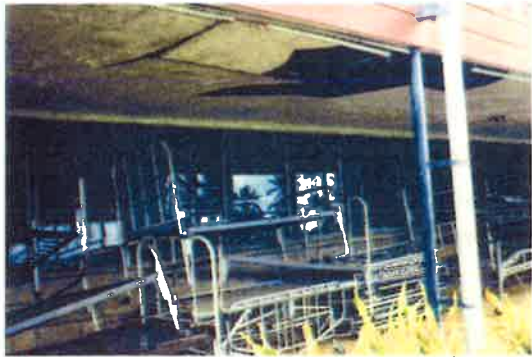
Obsolete beds cluttered under broken ceilings and leaking roofs were a common sight in the hospital in 1992
