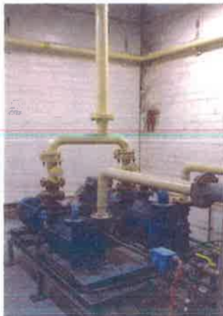
Figure 2 The pumps and housing at BHS
