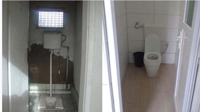
Through a $50,000 Rotary Foundation Global Grant, the Rotary clubs of Edwards, Colorado, USA, and Peja, Kosovo, brought clean water and new bathroom facilities to six area schools in Peja.
