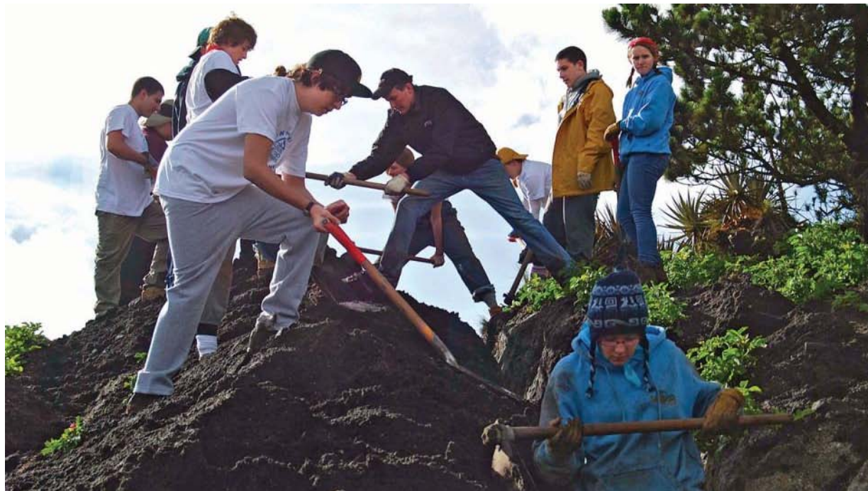
High school students from the Builders Beyond Borders program help install pipes that will carry water to the mountain town.
