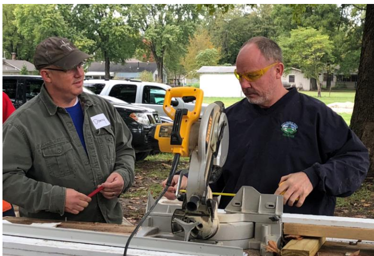
Danny Freeman (left) and Evan Holt measure and cut boards at the Habitat home in North Lawrence.
