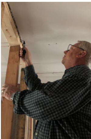
John Esau marks a section of sheetrock for the next step in construction.
