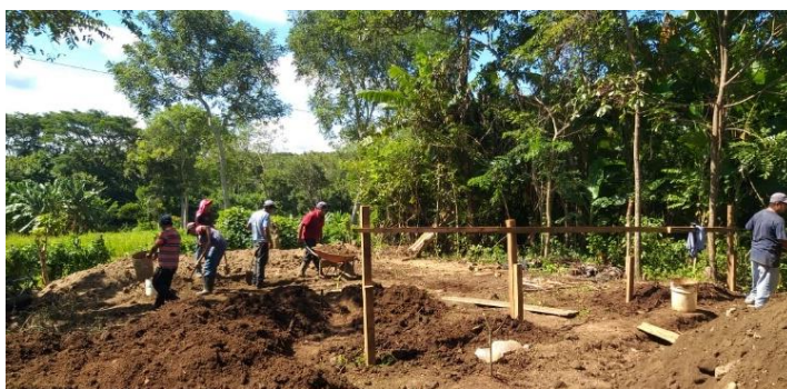
Prepping land for concrete slab for the retaining tanks Labor provided by the community
