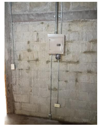
Completed wiring and control Panel in pump house
