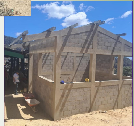
Workers pour concrete and lay block to prepare for the new community kitchen
