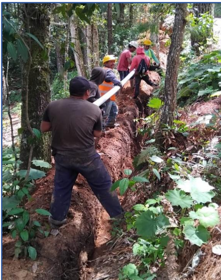
The project experienced some difficult trenching issues that were resolved using the community's volunteer manual labor to remove rock discovered just beneath the surface. Work began in 2025 and is 85% complete.
