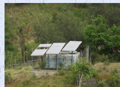
Solar pump at Boleha
