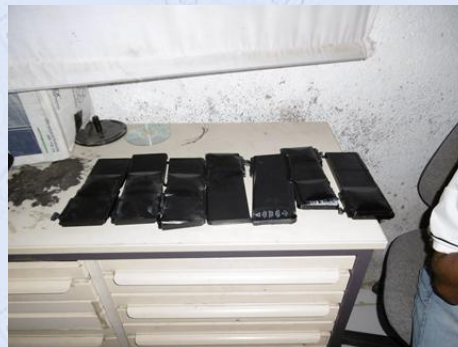
We lost 7 batteries on the way but all will still work
