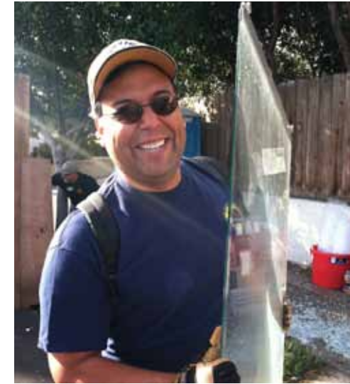
A large part of the Rotarian effort was clearing junk and trash from the property including old TV sets and a kitchen stove! Above, club President Steve Nuñez carries a glass shelf to a dumpster.
