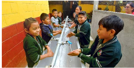
Handwashing station in a Guatemala School installed under WASH in Schools (WinS) grant
