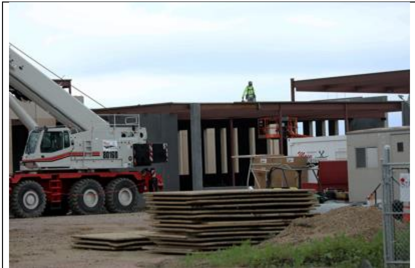
Contractors building the new Clay County Jail and Law Enforcement Center that will house the Vermillion Police Department and the Clay County Sheriff's Department are making progress despite some setbacks because of weather earlier this spring. David Lias/Vermillion Plain Talk
