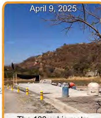
The 180 cubic metre septic tank is operational
