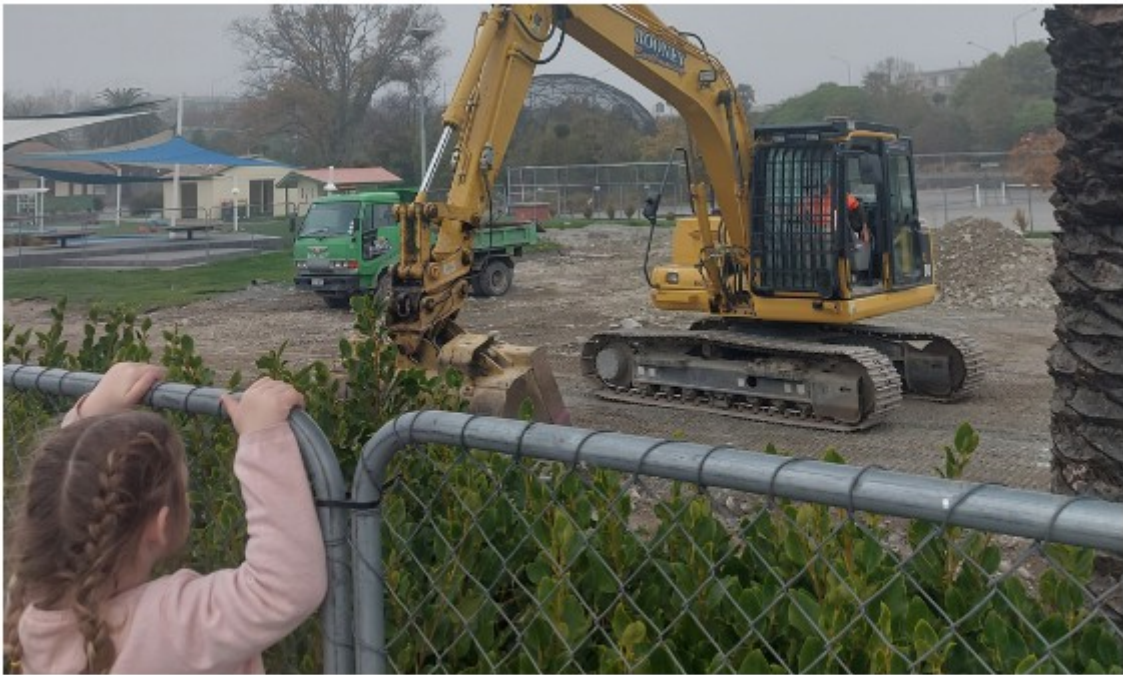
Annabelle Fauth, 4, watches the preparation work being done to be able to install the concrete curb.
