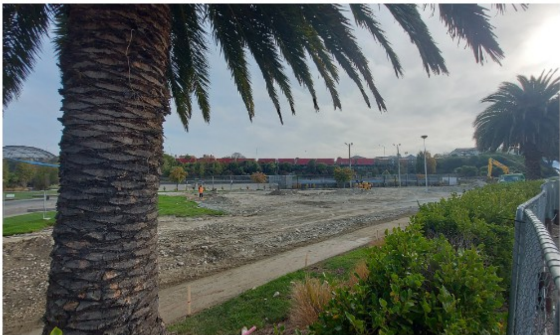
Here you can see a smooth surface prepared for the concrete curb. We are planning a rain garden between the Floor is Lava area and the hedge to help drain away storm water.
