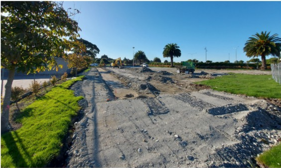
This area will soon be the flying fox. The first step was to scrape the topsoil away and backfill with river run. There's a concrete stormwater pipe that we have had to design the playground around which is in this area. So a lot of care has been taken to avoid damaging the infrastructure underground during the earthworks.
