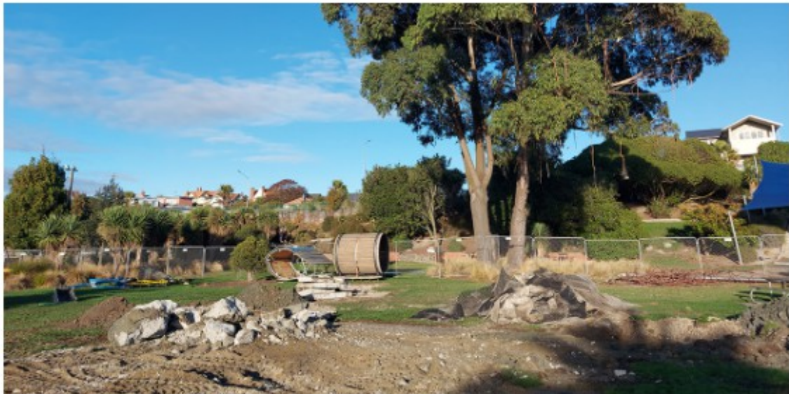
The rope pyramid and mouse wheel has been un-installed to relocate off site. Now that they are out of the ground we can assess their condition. The horse and mouse wheel have a few small issues which seem straight forward to remedy. The rope pyramid has some wear and tear which we are getting professional advice on.
