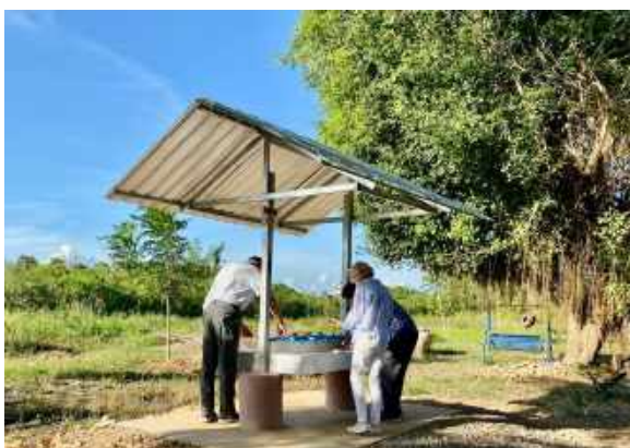
CFS builds hand washing and toilet facilities at government schools that have none.
