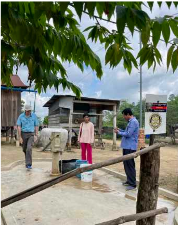
Communal water supply – bore and pump
