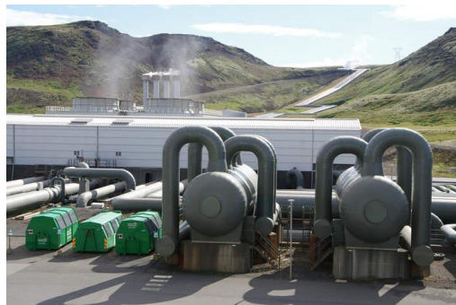
Hellisheiði geothermal plant.
