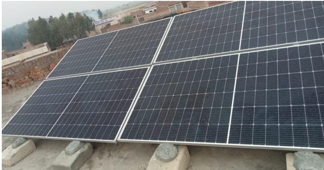
Solar Panels powering the water filtration plant
