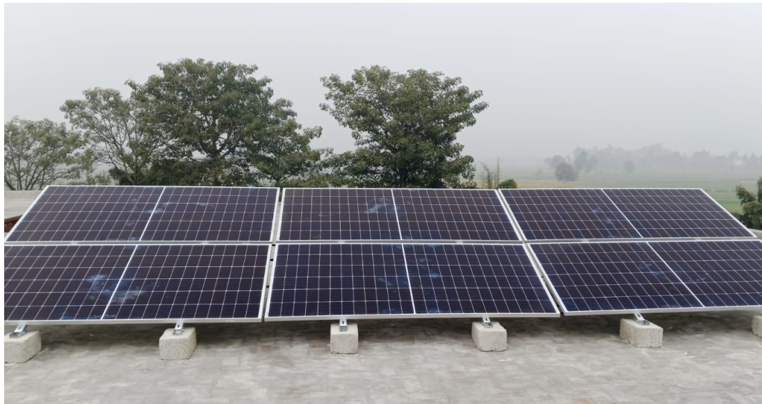
Solar Panels powering the water filtration plant
