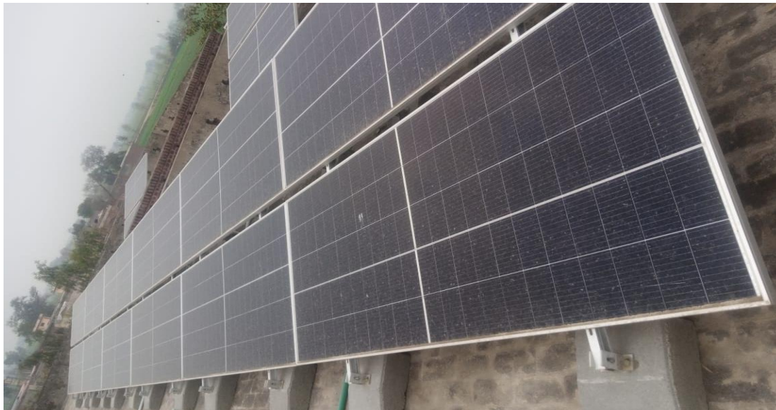
Solar Panels powering the water filtration plant
