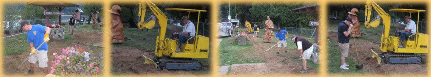
Rotarians installing wiring for the lights in The Hope Rotary Centennial Park
