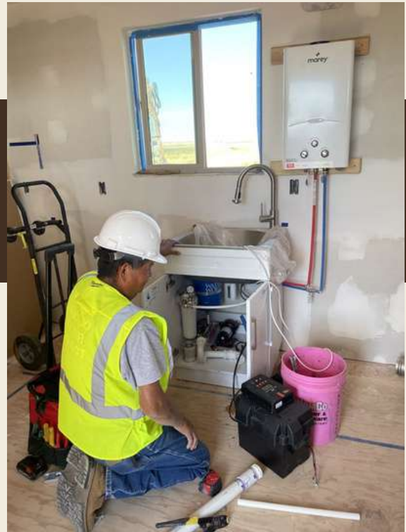
Cabinet w/ sink, pump, filter, baery, etc.
