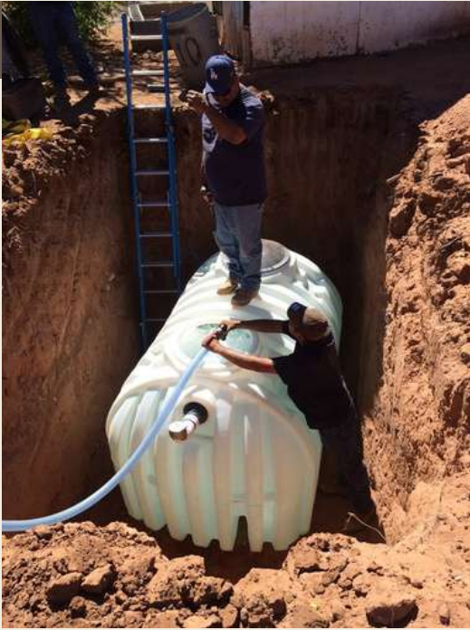
Buried 1,200 gallon water tank
