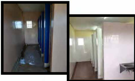
A toilet block at Khutliso Daniels Senior Secondary School (left) before the renovation and (right) after the renovation.
