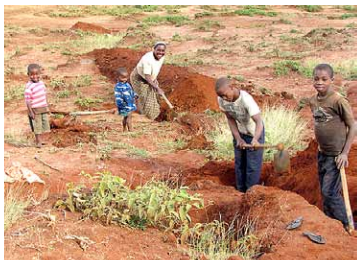
Villagers digging trenches for pipes from the water storage tank to distribution points in the village.
