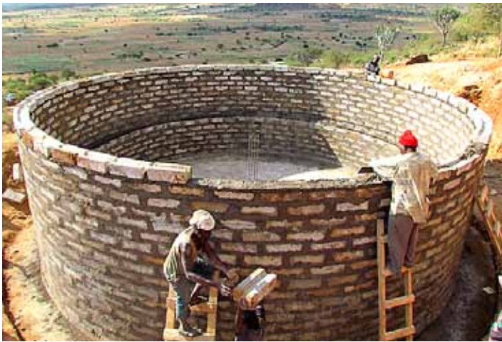
Villagers building the water tank under the supervision of the general contractor. Photos provided by Mary Wells/Ames
