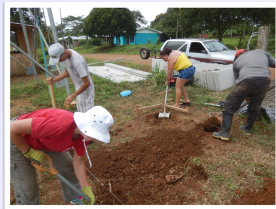
Digging holes at Combat well site for the chlorination treatment + mixing concrete by hand + installing concrete columns and first row of concrete panels = lots of heavy lifting!
