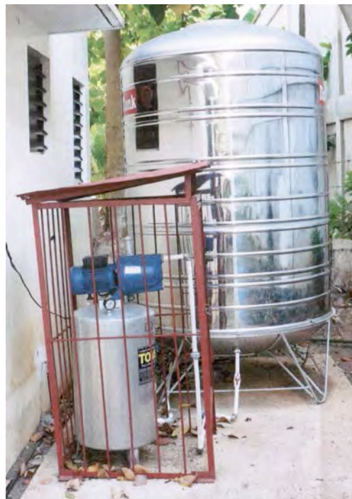
Stainless Steel Water Tank and the Pressure Pump on the concreted base
