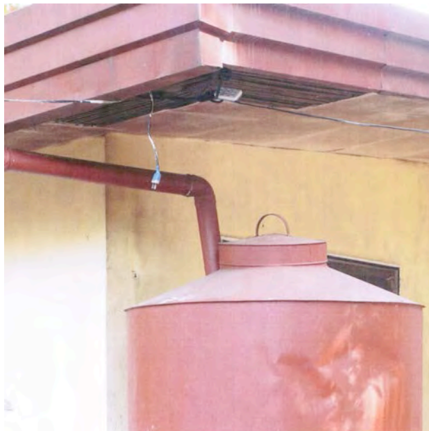
Repositioned water catchment tank with repaired gutters to cater for the House of Hope & the Annex
