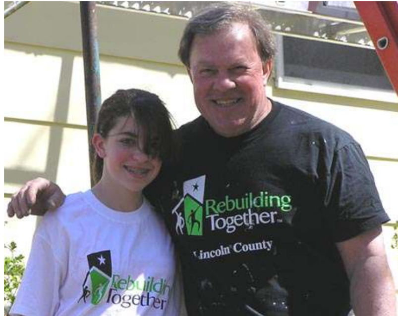
While Rotarian Bill Bailey roofs, his daughter Christin paints, and they both wear the results. Rebuilding Together has a job for all ages and skill levels.
