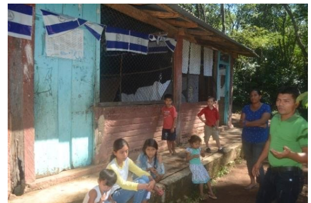
Due to frequent seismic activity in Nicaragua, the entire structure in El Papalón is vulnerable to failure and collapse.
