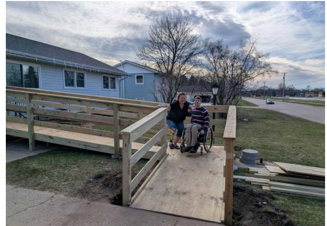
Berlin Rotary Club members construct a wheelchair ramp for a community member.
