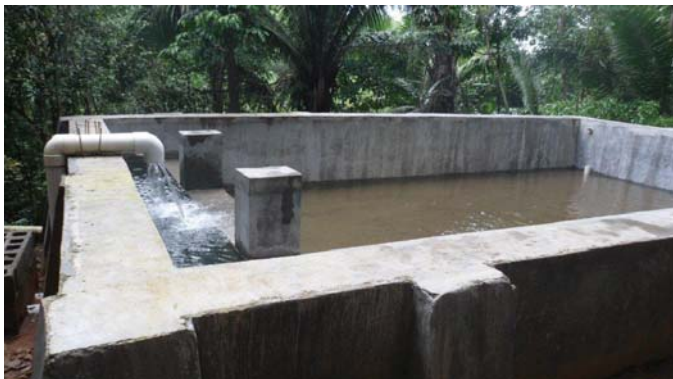
The Buenos Aires sediment settlement/ slow sand filter tank providing clean water for 424 families
