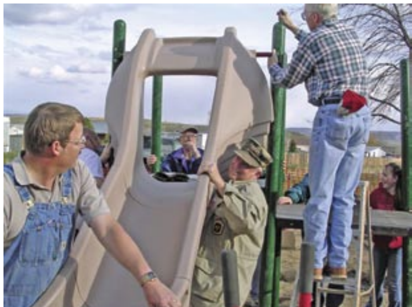
Members of the Rotary Club of Craig (Moffat County), Colorado, USA (D-5440) building a playground in their own community for low-income families.
