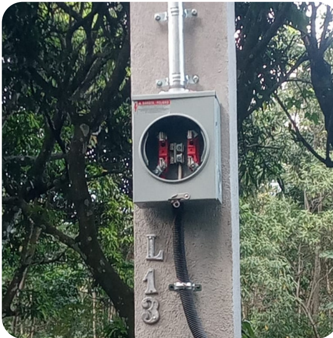
National electricity grid connection box
