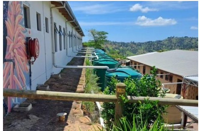
Some of the water tanks installed at Philakade ensuring continuous water supply to the facility. A borehole has also recently been installed.
