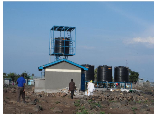
Water tanks on the island.
