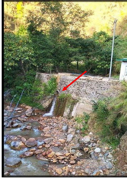
Figure 1 - Discharge port / outlet (see red arrow) of the spring water that flows out to the Baguio Gold creek below it.
